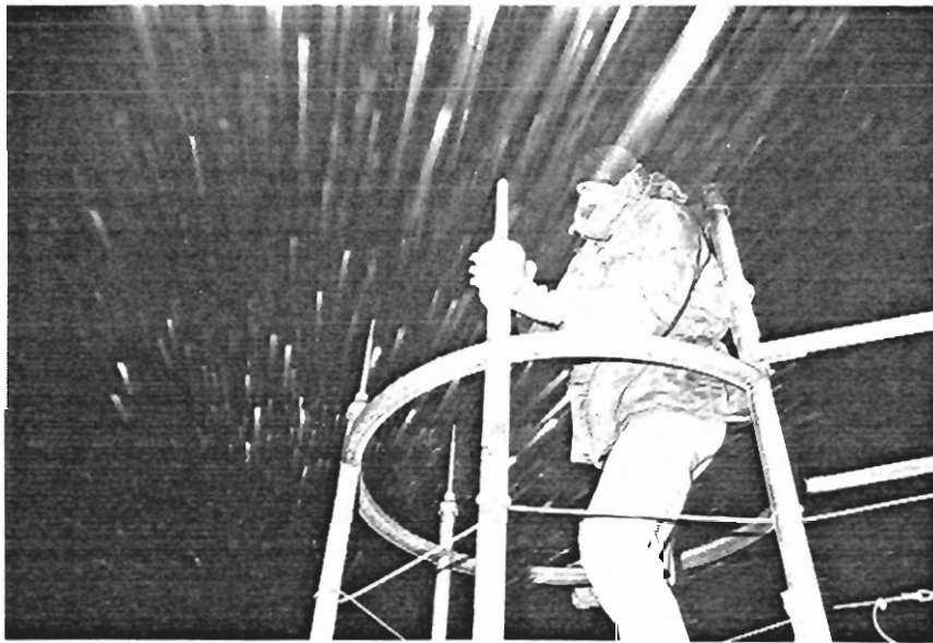
Figure 5: Chuck Franklin of Franklin Engineering installing his pneumatically deiced wind and ice probe on the tower superstructure. Two D. N. E. ice detectors are also visible.
