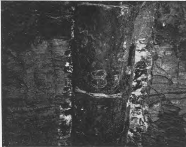
FIGURE 8 — Photograph of excavation in frozen silt showing refrozen soil and ice around a steel pipe pile without use of artificial refrigeration.
