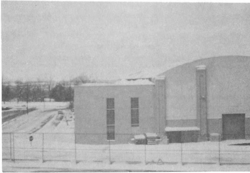
FIGURE 7 Snow Sliding Off Arched Roof
