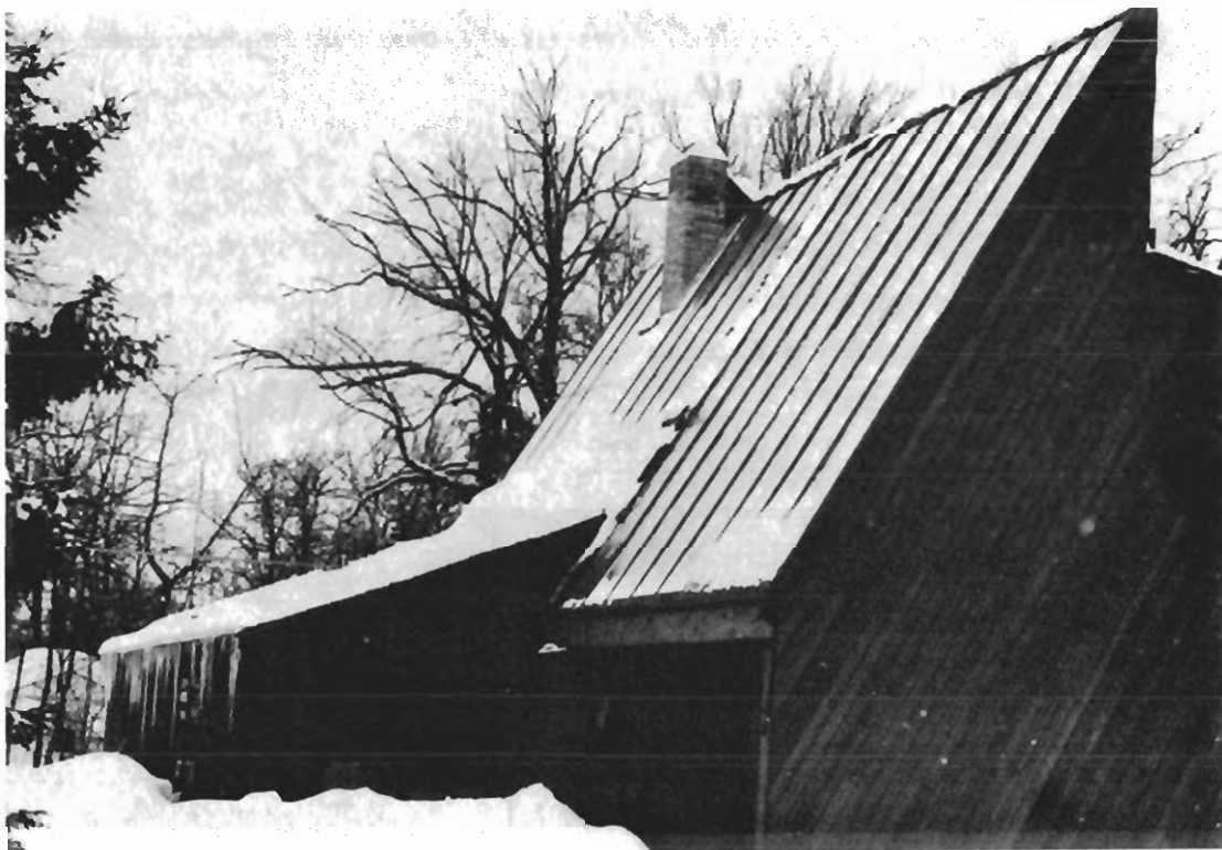
Figure 7: Obstruction below Steep Collectors
